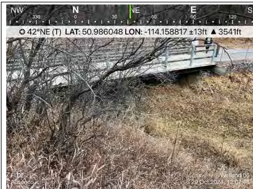
Photo 123 View north from FL-02 inflow site. Photo taken during fall sampling on October 29, 2024.
